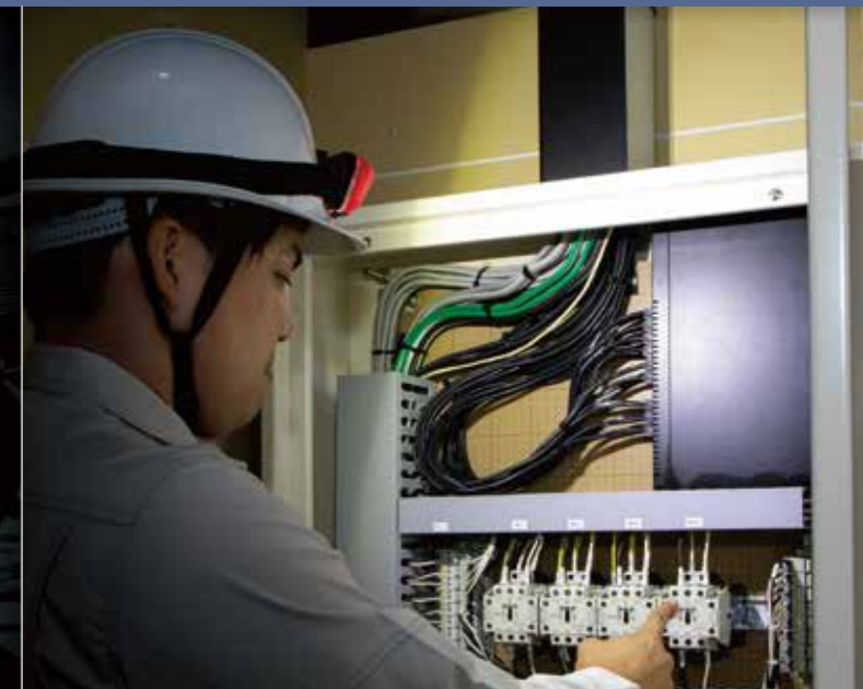
For inspection of the switchboard
