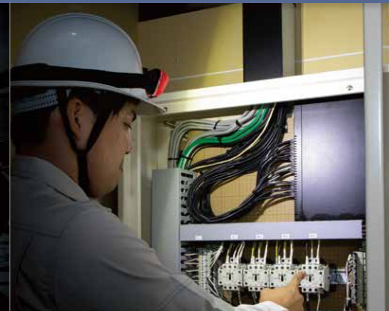
For inspection of the switchboard
